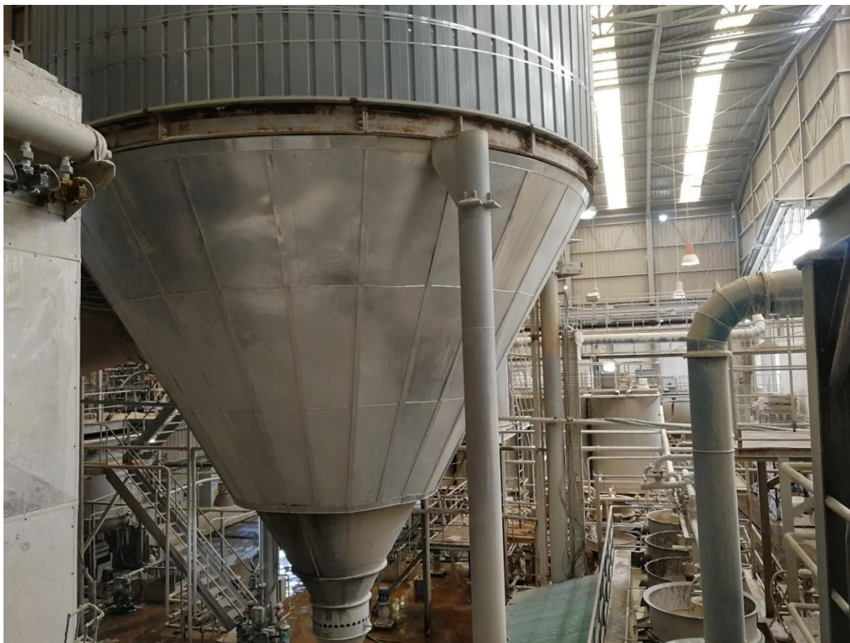
Figure 1.3 - General view of preparation unit
