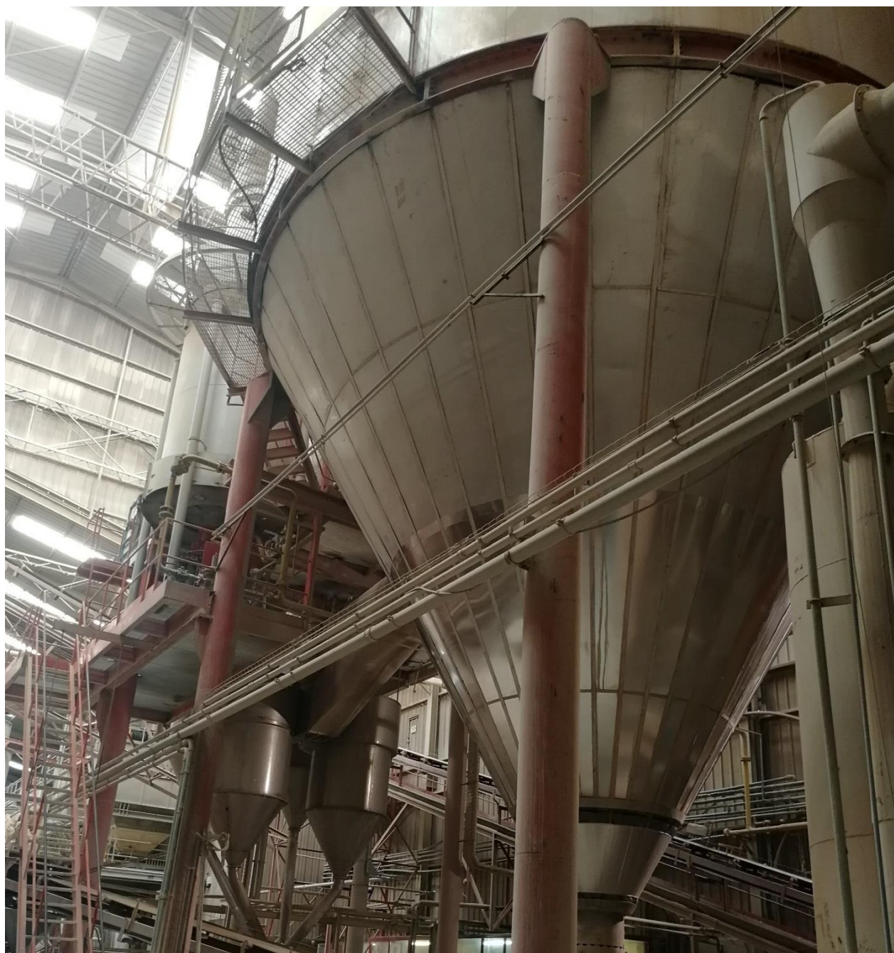
Figure 1.3 - General view of preparation unit
